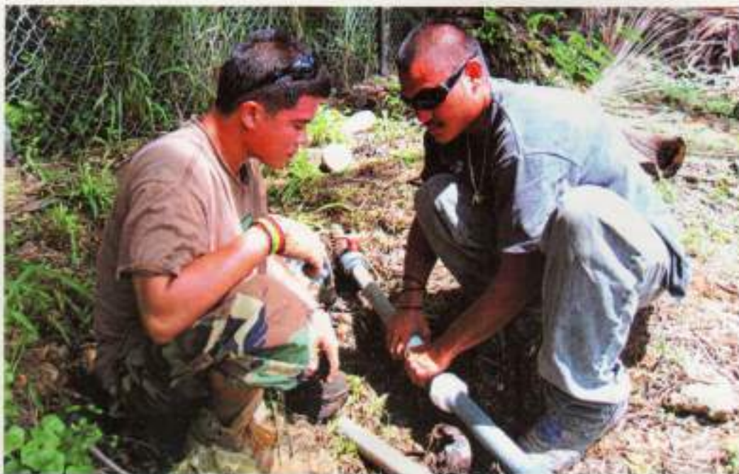
CUC Water & Wastewater Division Trade Assistants, Patrick Blas & Peter Attao, repair leaking water line
