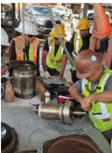
CUC Saipan Water & Wastewater
