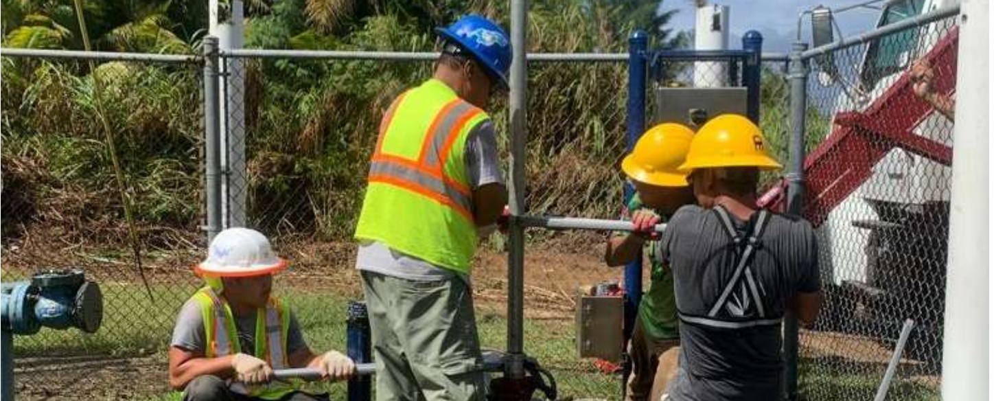
Rota Water Operators Jimmy Atalig Jr., Anthony Barcinas, Austin Lizama, and Darien Rangamar install the pipe for one of the three deep wells on Rota. The wells can be used as a back-up to the primary water source from the Main Cave.
