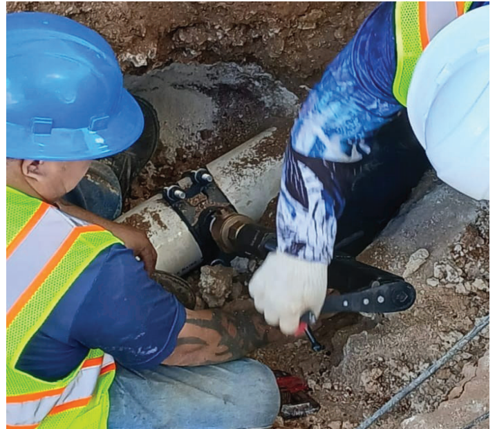
CUC Rota Water Operators Pete Taitano and Poly Jon Manglona install a corp stop—a key valve linking new service lines to the main water supply—helping ensure clean, reliable water for the island.
