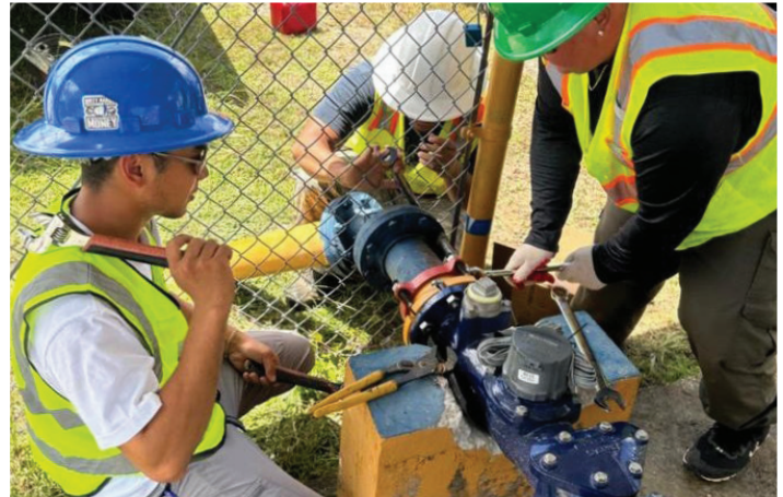
CUC Rota water operators Austin Lizama, Pete Mendiola, and Kurt Maratita install a new flow meter to help improve water system monitoring and reliability.
