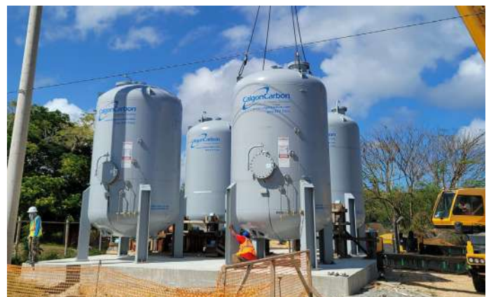
Four (4) Granular Activated Carbon Water Filtration Systems being installed for the Isley Field to remove PFAS from the water.
