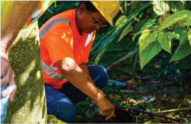
CUC Saipan Water Distribution Operator Specialist, Julie Camacho, installing a temporary water meter.
