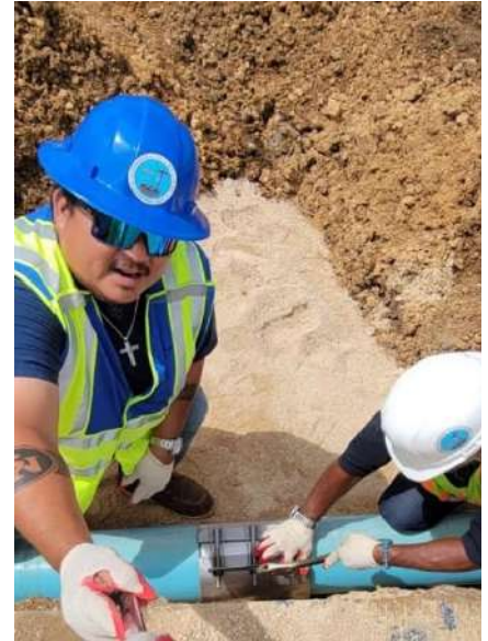
John Sablan and Laurence Tumed repair the main waterline in Marpo Heights II
