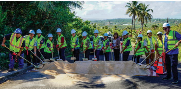
CUC remains committed to delivering safe, reliable, and sustainable water services for its customers across the CNMI. As part of this commitment, the groundbreaking ceremony for the Carolinas Heights Waterline Replacement Project in Tinian marked a key step in upgrading critical infrastructure to support current and future water needs.
