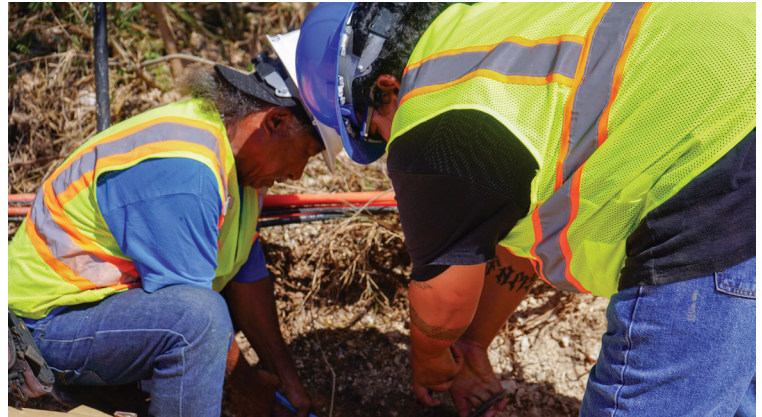
CUC Tinian water operators work daily to ensure safe and reliable water service for the island community—conducting system checks, performing maintenance, and keeping the water flowing. Here, Laurence Tumed and John Sablan are hard at work in the field.
